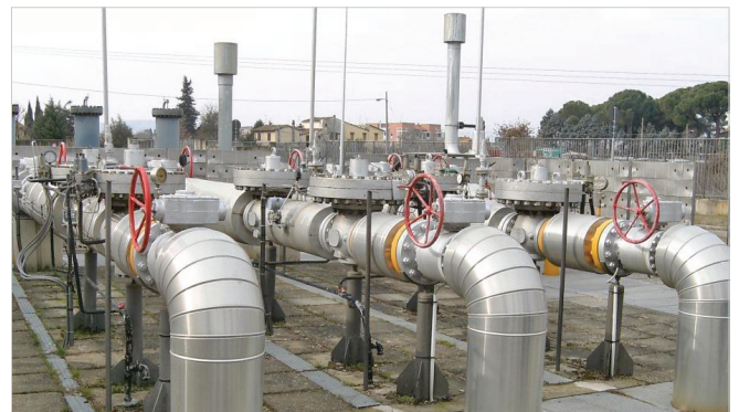
Toscana Energia City Gate before upgrade - 6" Top Entry Regulators without Integrated Silencers - With wall panels & pipe insulation
