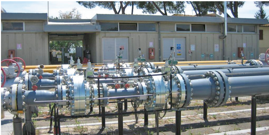
6" FL Wide-Open Monitors and 6" FL/SRS Regulators installed in Toscana Energia City Gate, Ugnano Florence, Italy
