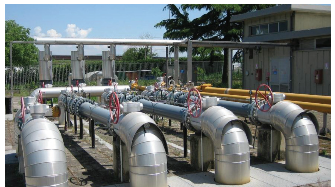
Toscana Energia City Gate after upgrade - 6" FL Axial Flow Regulators with Integrated SRS Silencers - Without wall panels and pipe insulation
