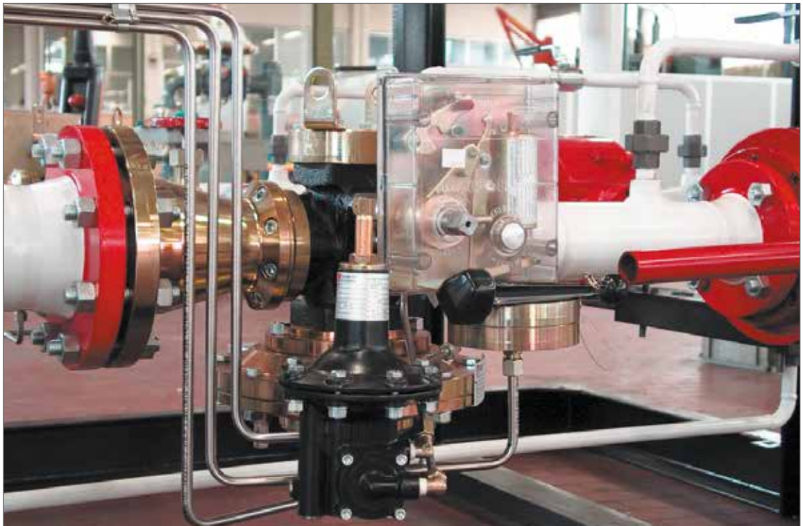
Detail of reducing unit with CB-SRS. Right to left gas flow
